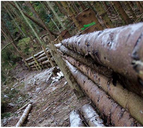
A large timber dam forming one part of the Slowing the Flow project near Pickering. Yorkshire visit 6 th December 2011.
